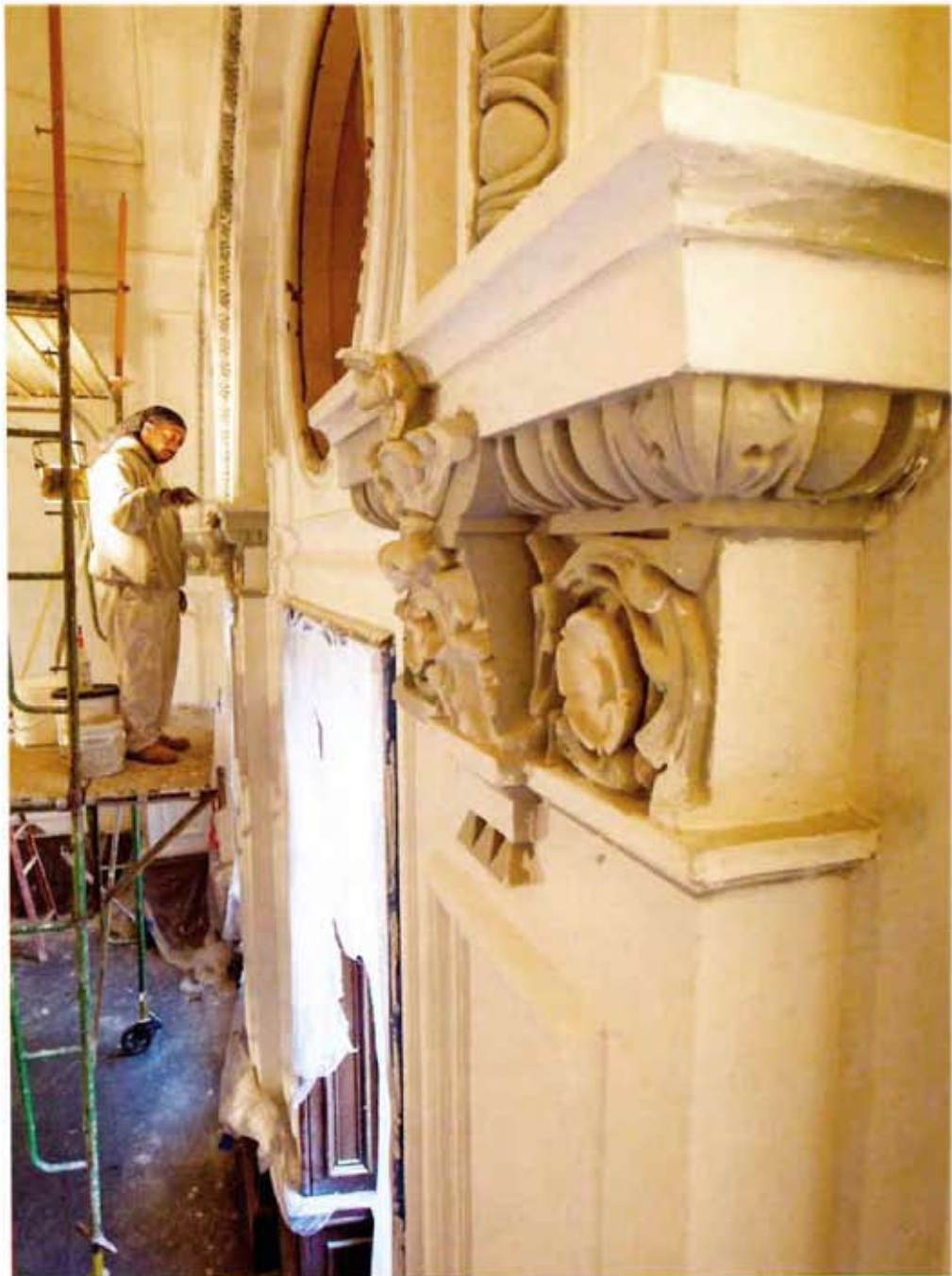
Details. Anthony Riley works on the damaged decorative plaster molding in Columbia City Hall.
